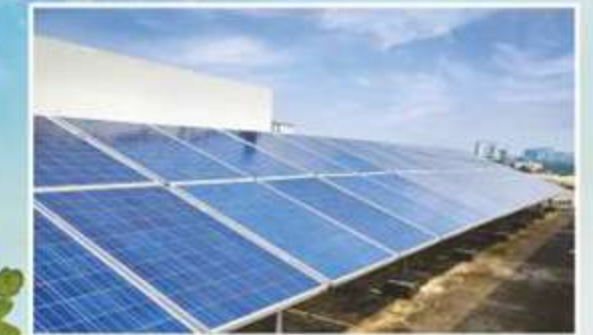
A Green Initiative - 40 kW Grid Connected Solar PV Rooftop Plant on the Corporate Office of WBPDCCL
